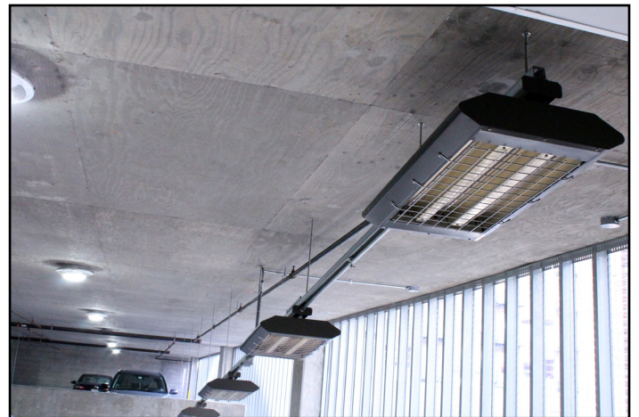
Infrared heaters installed in JeffJack parking garage using standard mount
