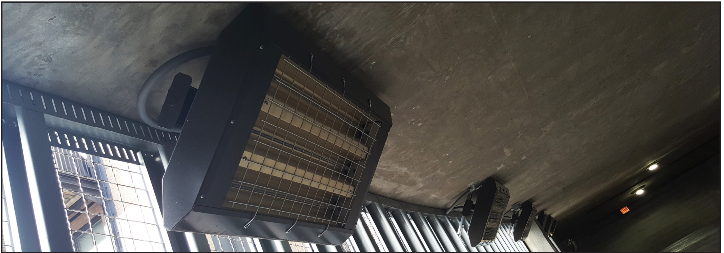
Berko infrared heaters mounted on side wall in the JeffJack parking garage
