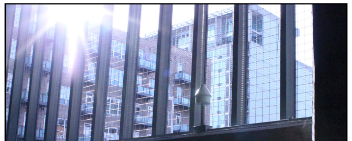
A small white sensor connected to the infrared heaters detects moisture and temperature
