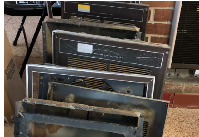
Building's Original Wall Heaters (Prone to poor/unsafe air quality)
